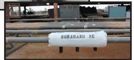
HB Insulator Wrap installed on center wear pad
